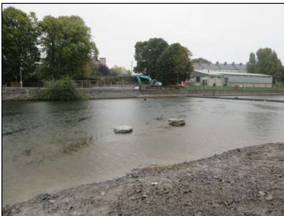
Plate 2 The River Nore at the location of the new bridge. Two structures have been constructed within the river. The riverbed in this part of the river has been significantly altered.
